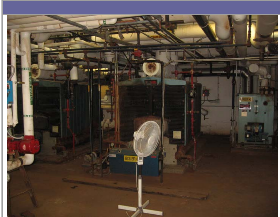
View of mechanical room
