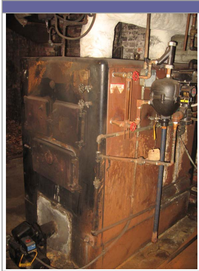
View of the boiler
