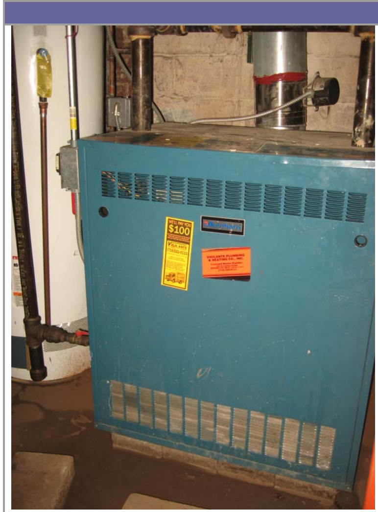
View of the boiler
